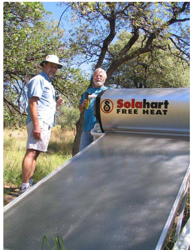
John Weiss and Drum Haverstock inspect the new solar hot water heater.
