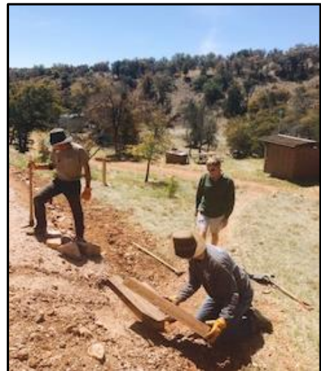
Installing new steps adjacent to the new roadbed on the path to the caretaker trailer.
