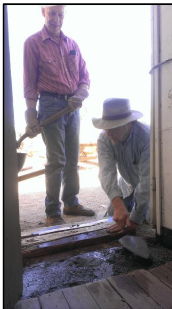
Pete van Cleve and John Weiss pour concrete footing for door threshold. June 14, 2014 volunteer day. (Photo courtesy of Mark Doumas)
