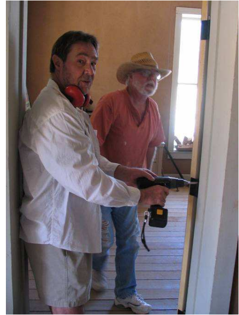
John Weiss and Drum Haverstock install one of many Headquarters Building doors
