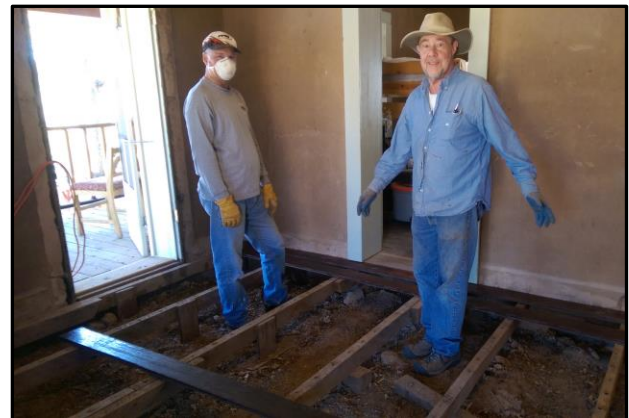
Ron Parrish and John Weiss finish removing floor boards in the living room.
