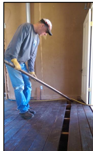
Ron Parrish finishes placing refurbished floor boards in the living room of the rental cabin.
