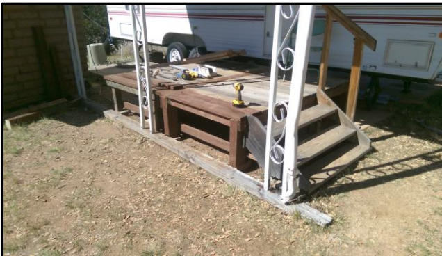
Caretaker Steve Waylett rebuilt the porch on the caretakers trailer. The final product even has railing all the way around the porch.
