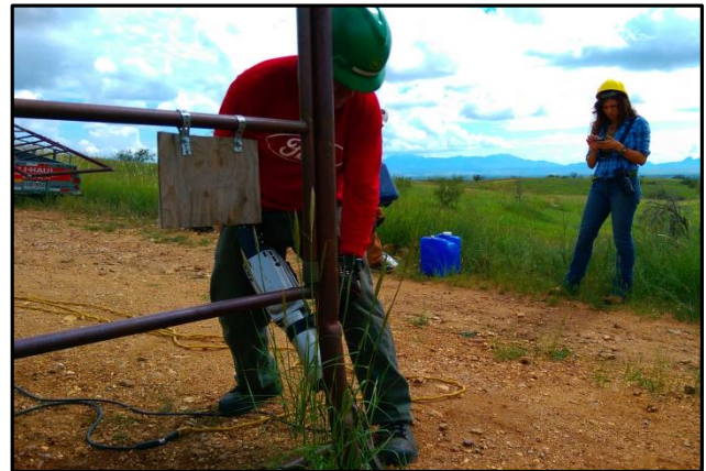
Removing the north gate required the use of a pneumatic hammer. (Photo courtesy of Mark Doumas)
