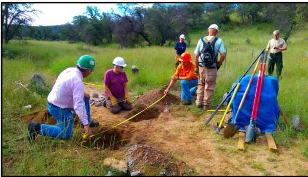
After removing the old south gate, careful measuring is required. (Photo courtesy of Mark Doumas)
